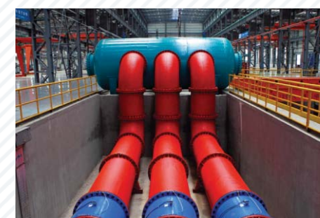
Testboard for large and medium-sized pumps
