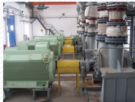
BB2 Process Pump in Urumqi Petrochemical Company
