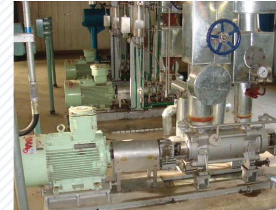
Sulfur Recovery Facility in CNPC Shijiazhuang Branch
