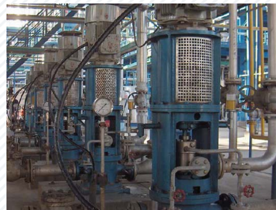
20,000 tons / year MaleicAnhydride Plant in Lanzhou Petrochemical Company
