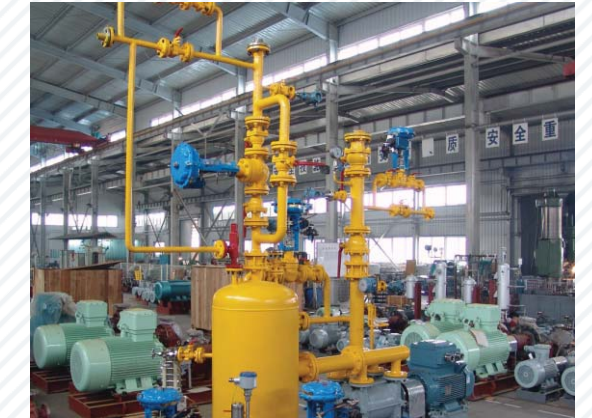
Vacuum Pump System Site
