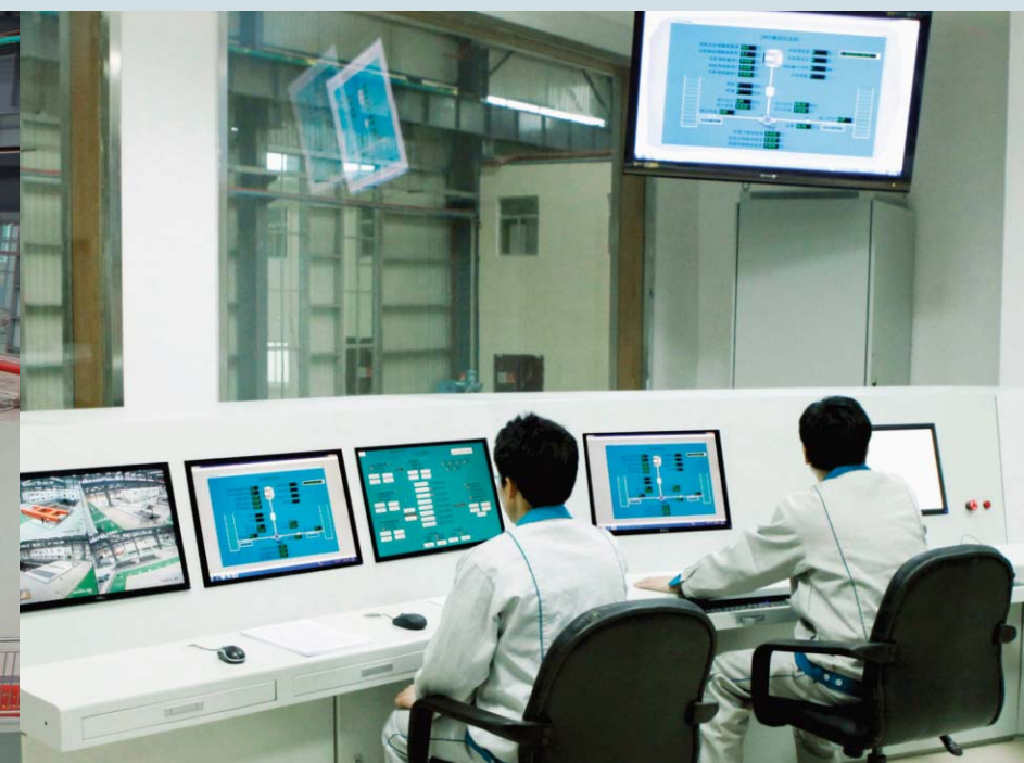
Central Control Room of Host Computer in Test Station
