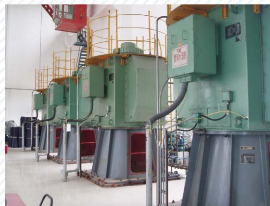
Huadian Yuannan Zhenxiang Power Station
