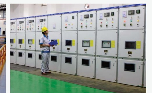
Electric Control Room in Test Station
