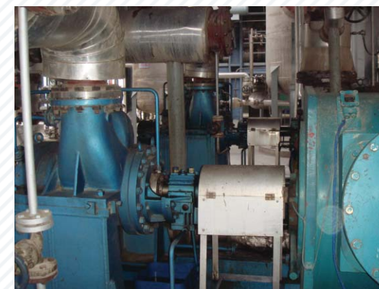
BB2 Pump in Xinjiang Jinhuyang Chemical Co., Ltd.
